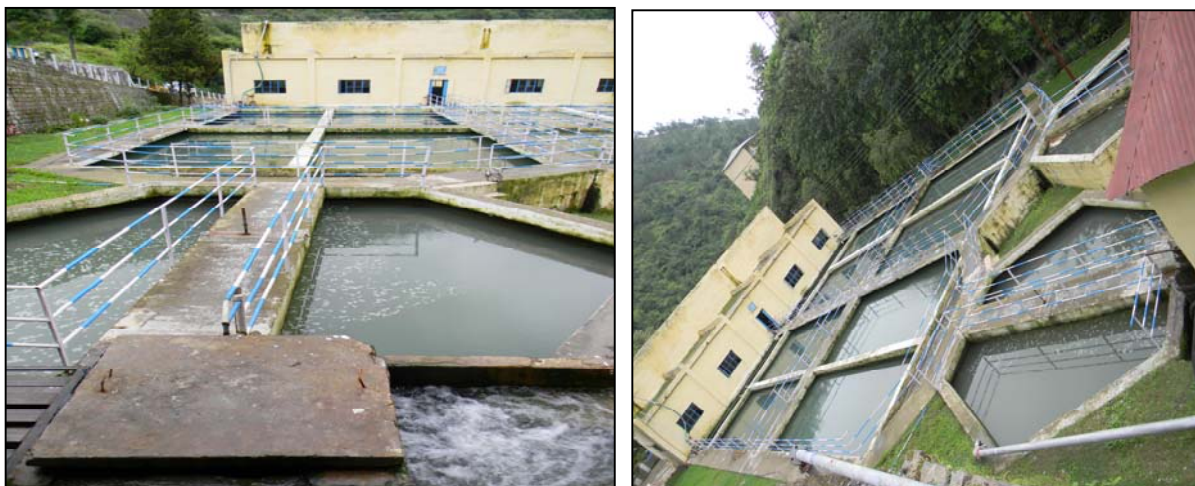
Fig. 31: A View of Ashwani Khad Water Treatment Plant in the Study Area
