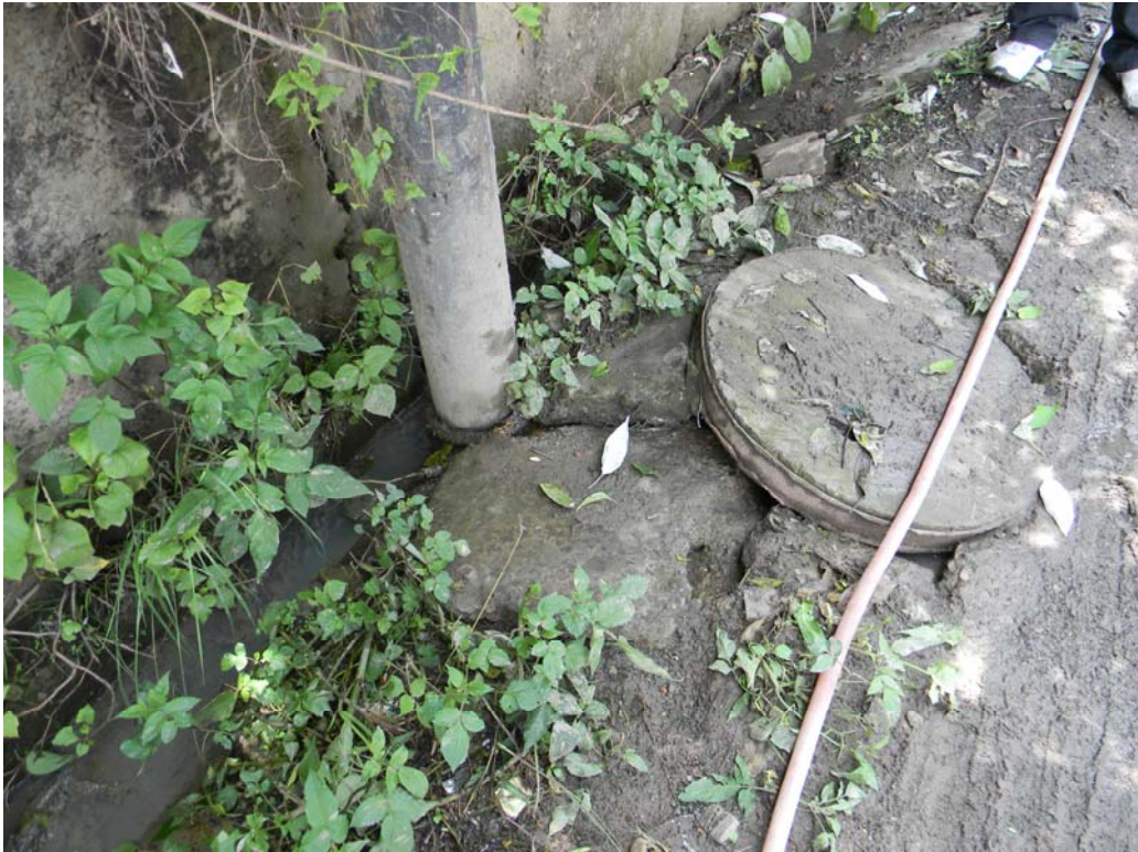
Fig. 14: A view of Manhole Overflow in the Study Area
