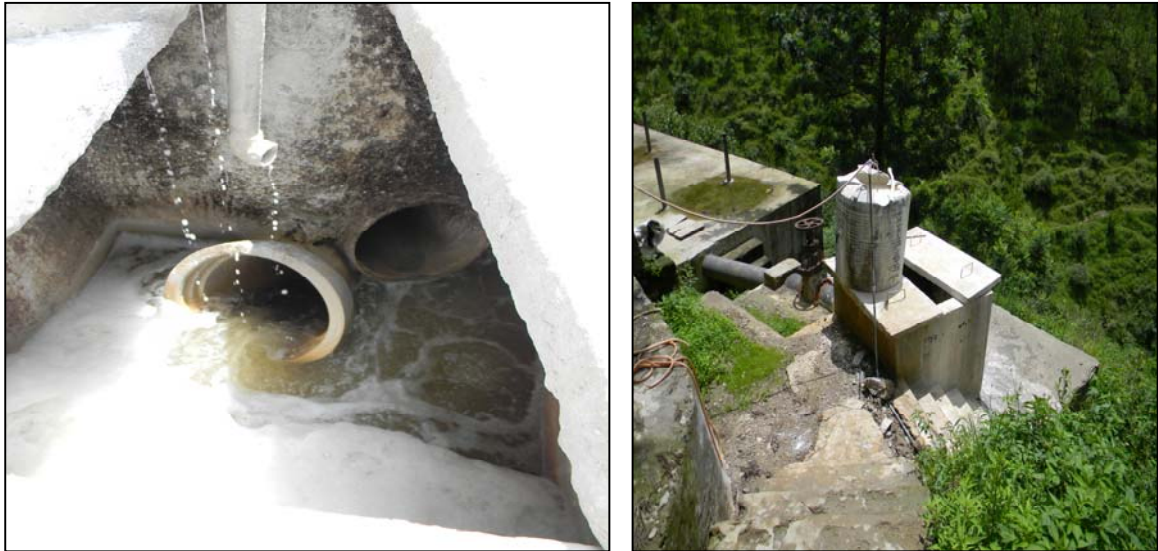
Fig. 27: A View Showing Hypochlorite Dosing System
